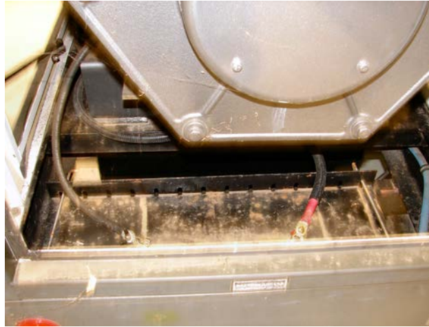
Figure 50B-7: 5080DE Aircraft Air-conditioning Battery Bay
