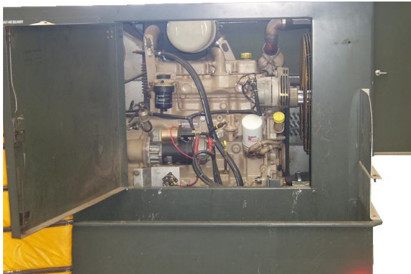
Figure 50A-6: TEC 300 AC Aircraft Air-conditioning Unit Condenser Engine
